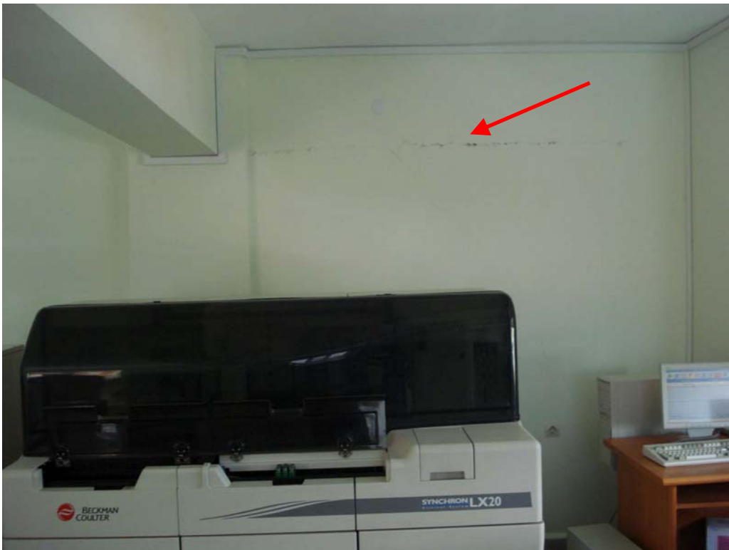
Figure 68: Hospital building, completed in the beginning of 2000's, biochemistry lab. (same room) , machine has displaced, and infill wall cracked during earthquake
