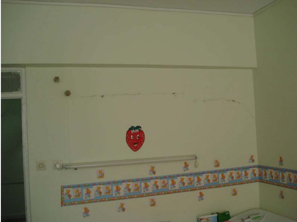
Figure 69: Hospital building, completed in the beginning of 2000's, infill wall crack
