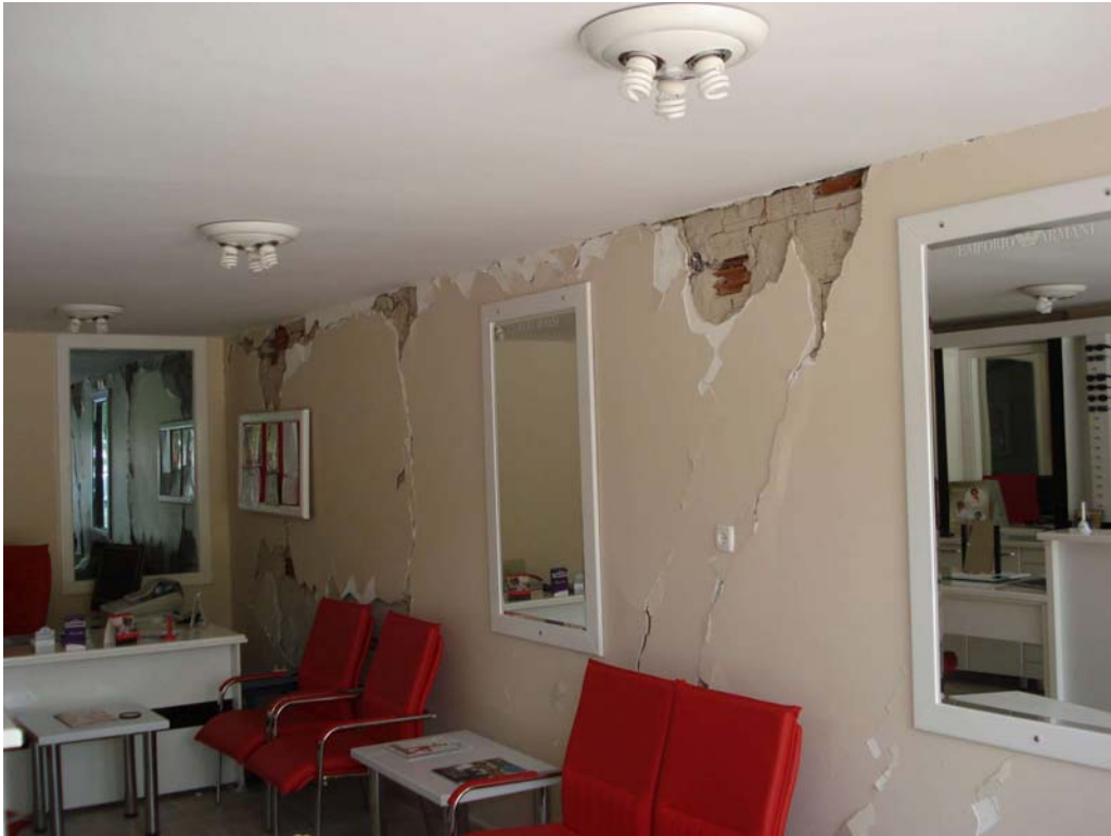
Figure 73: Building next to hospital complex – staircase infill wall cracks, spalling of plaster (ground floor, being used as pharmacy and optician)
