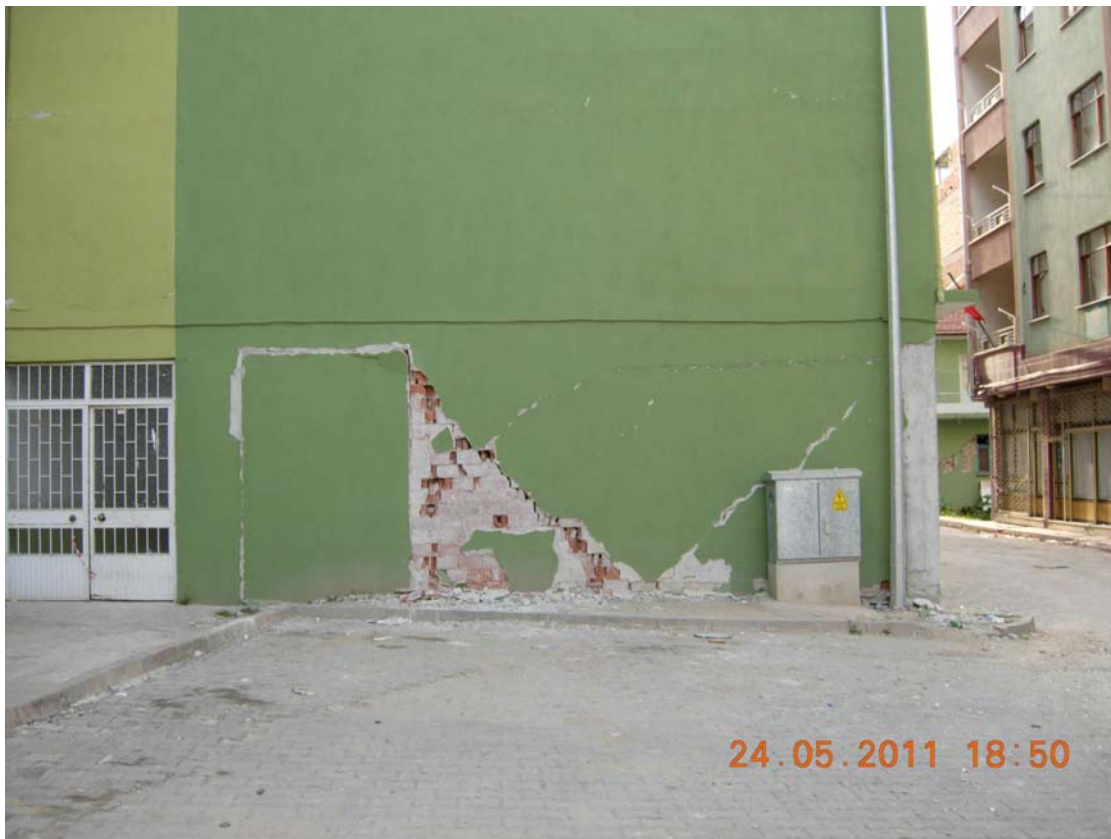
Figure 56: Damaged building, in front of the collapsed building, cracked infill wall at side
