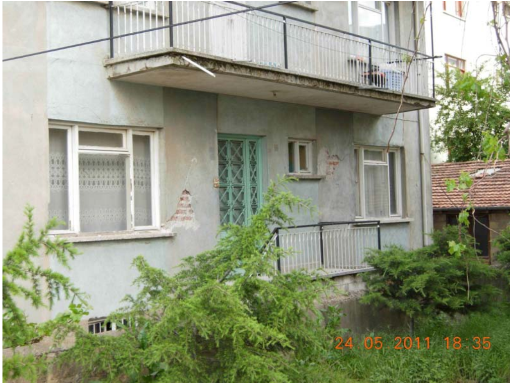
Figure 83: Spalling of plaster on ground floor of 3 storey brick masonry building
