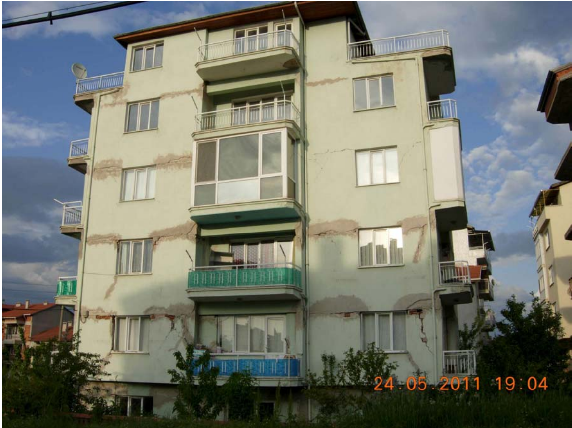
Figure 57: Damaged building, which was apparently damaged during previous earthquakes, plaster was repaired, but same locations cracked again in this earthquake
