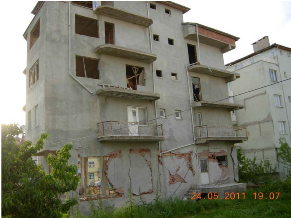
Figure 58: Non-structural infill wall damage on a new building which is still under construction
