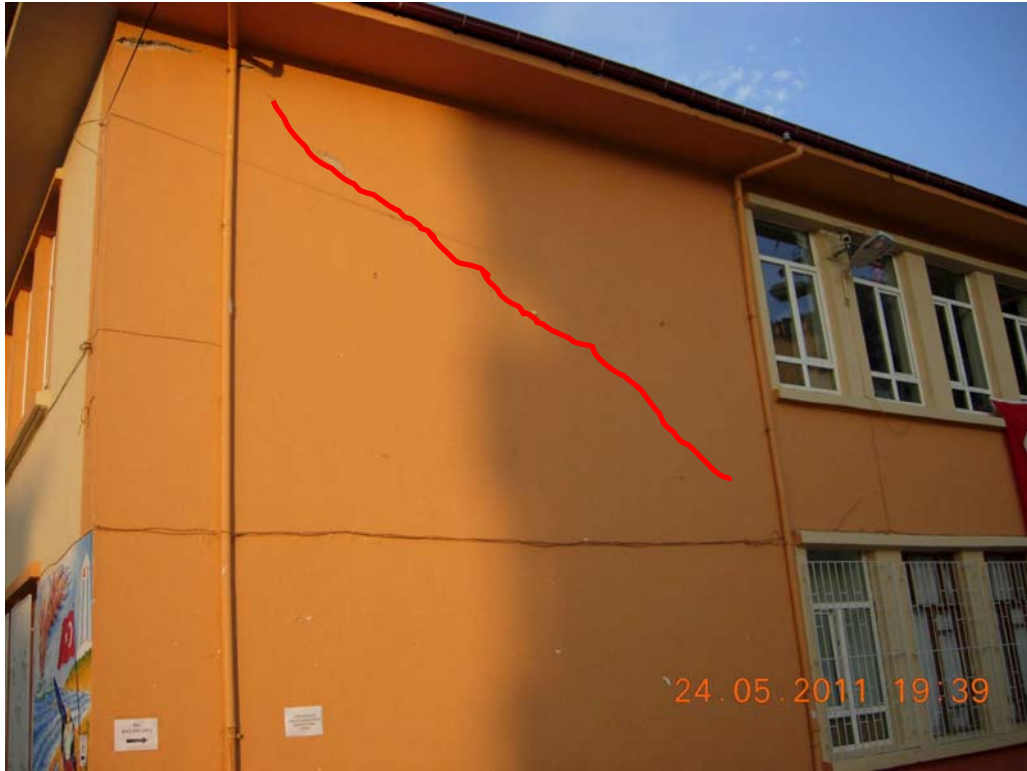
Figure 77: Cracks on outer walls of masonry part of the school building, 2nd floor
