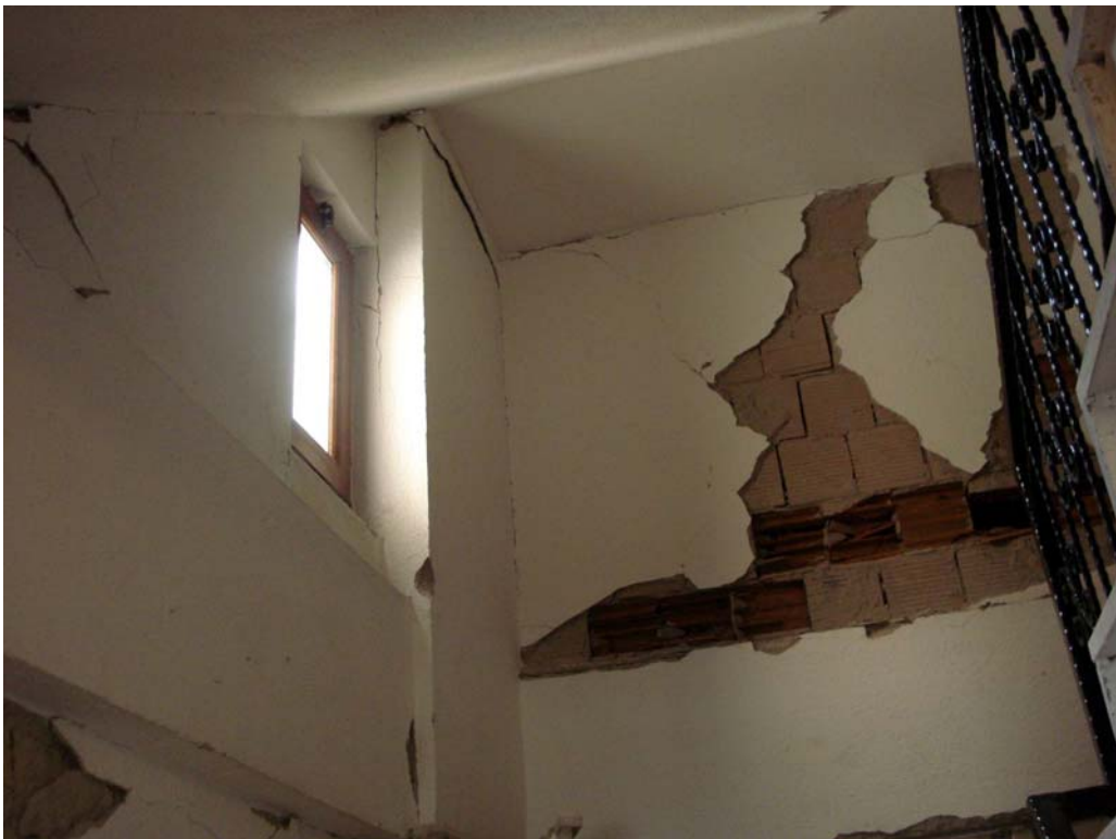
Figure 72: Building next to hospital complex – staircase infill wall cracks, spalling of plaster
