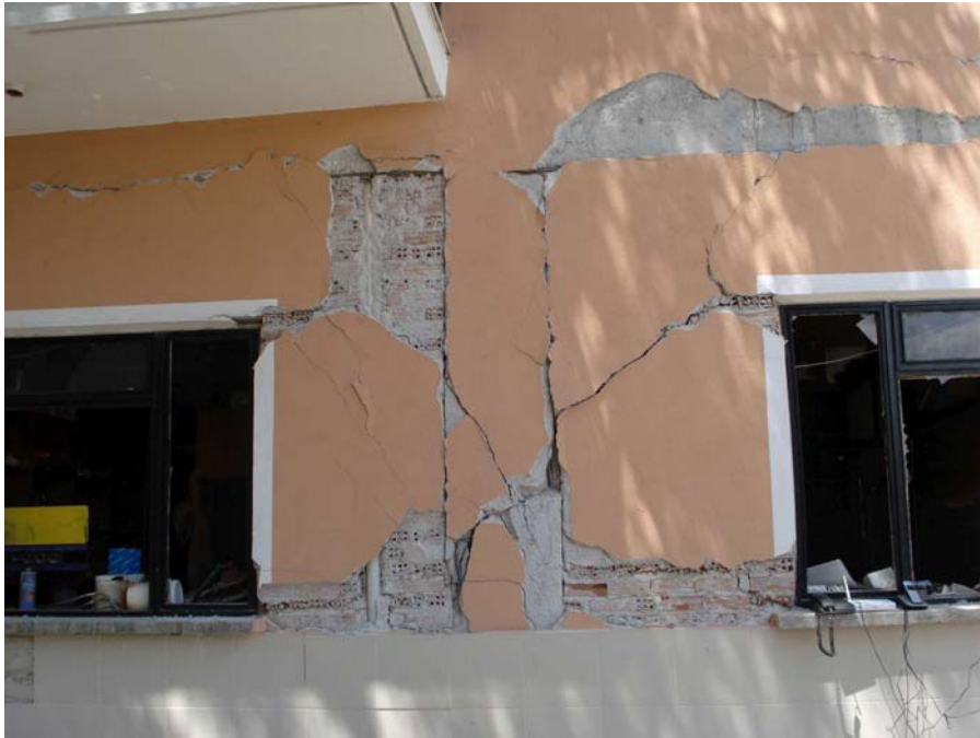
Figure 52: One of few examples for heavy structural damage, column behaved as a short column ,infill walls were composed of fired structural bricks instead of standart infill wall bricks.
