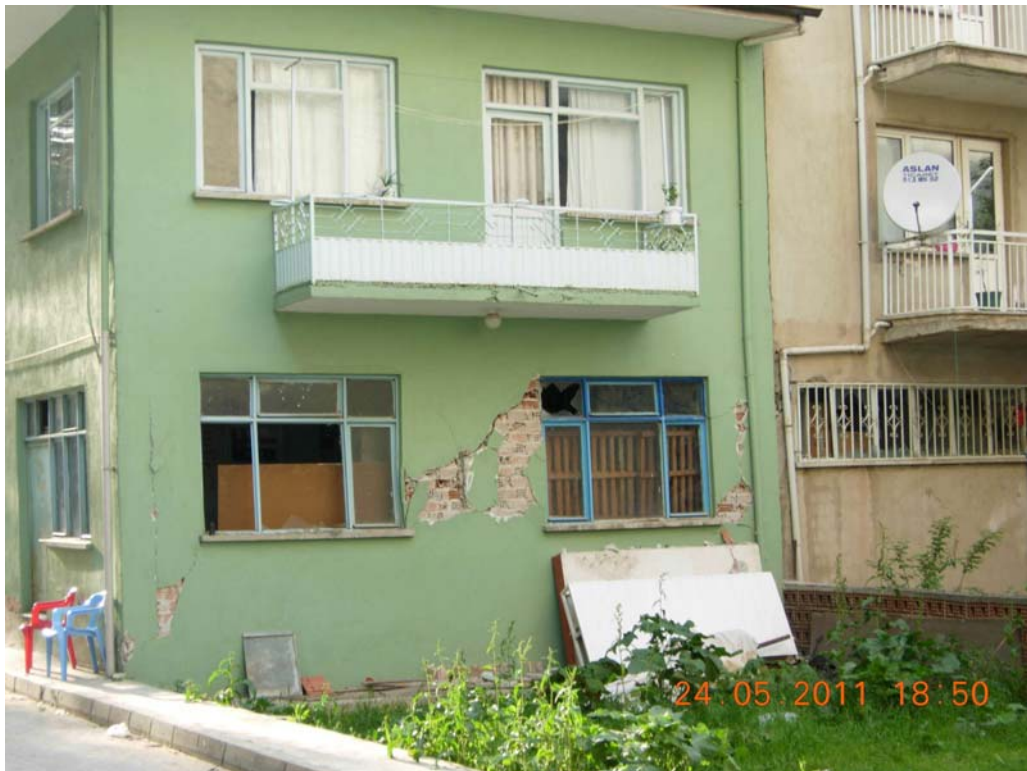
Figure 84: Spalling of plaster on ground floor of 2 storey brick masonry building
