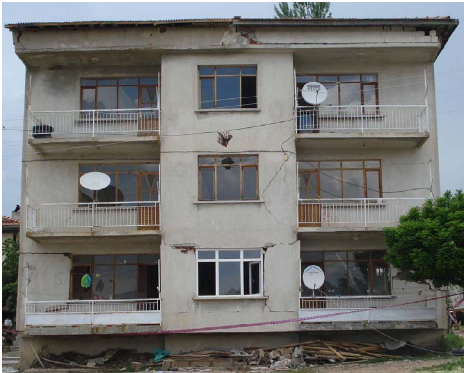
Figure 80: Gökçeler village, grade 3 damaged building, front view
